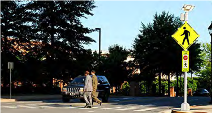
An example of a solar powered crossing signal.
