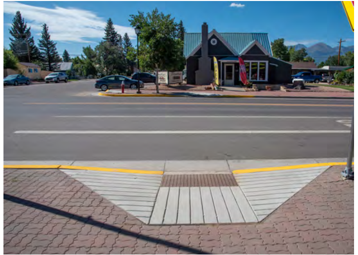
ADA ramps with grooves parallel to the walking direction are difficult for wheelchairs to navigate.
